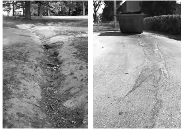
Left, clear evidence of severe erosion from stormwater runoff at Thoreau Elementary; right, a leaking garbage dumpster at Cherokee Middle School.
