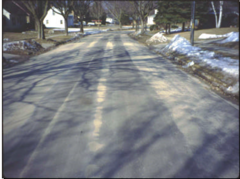
Road Salt and Sand Accumulation
