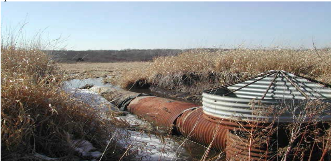
Breached storm water detention facility (Pond #4) in South East Marsh.
